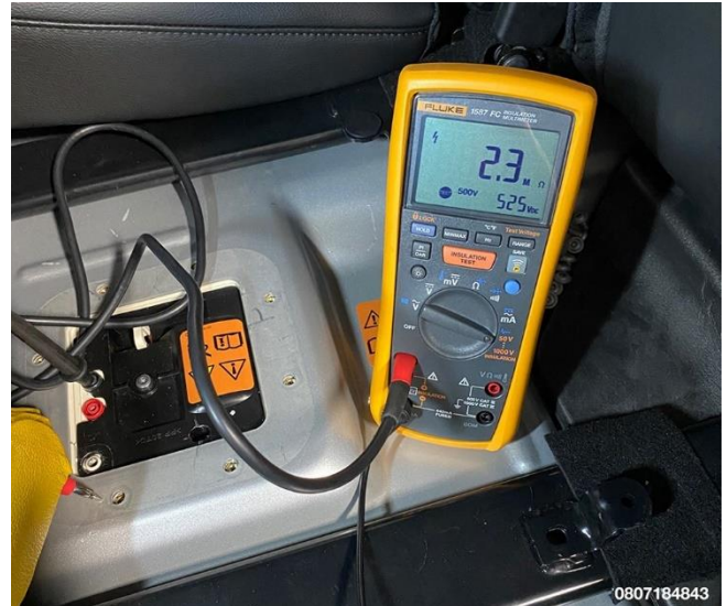
Figure 38 – Measure and Record Isolation Resistance Between HV Negative Test Point and Chassis Ground
