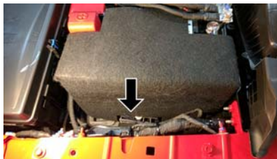
Auxiliary Switch Connections – Under Hood
